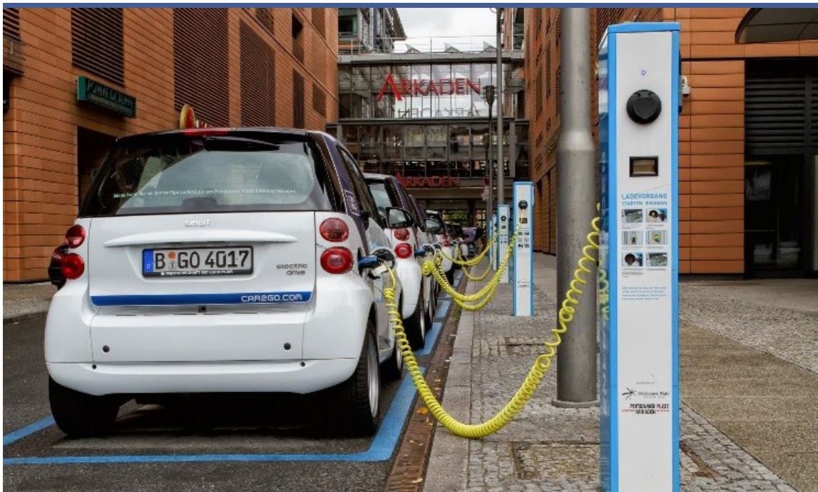
M-3.4: Install E-Vehicle Chargers
